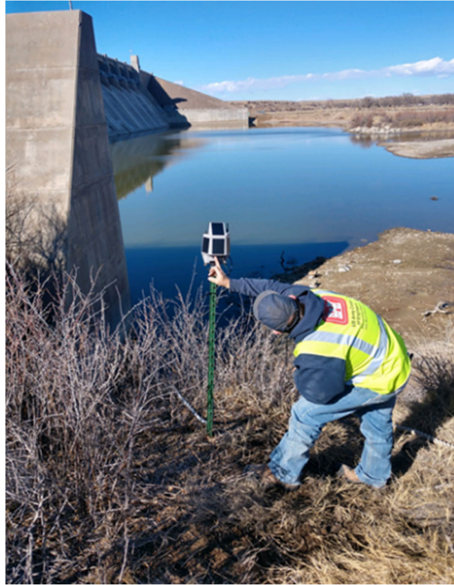
Flood sensor installation at John Martin Dam
