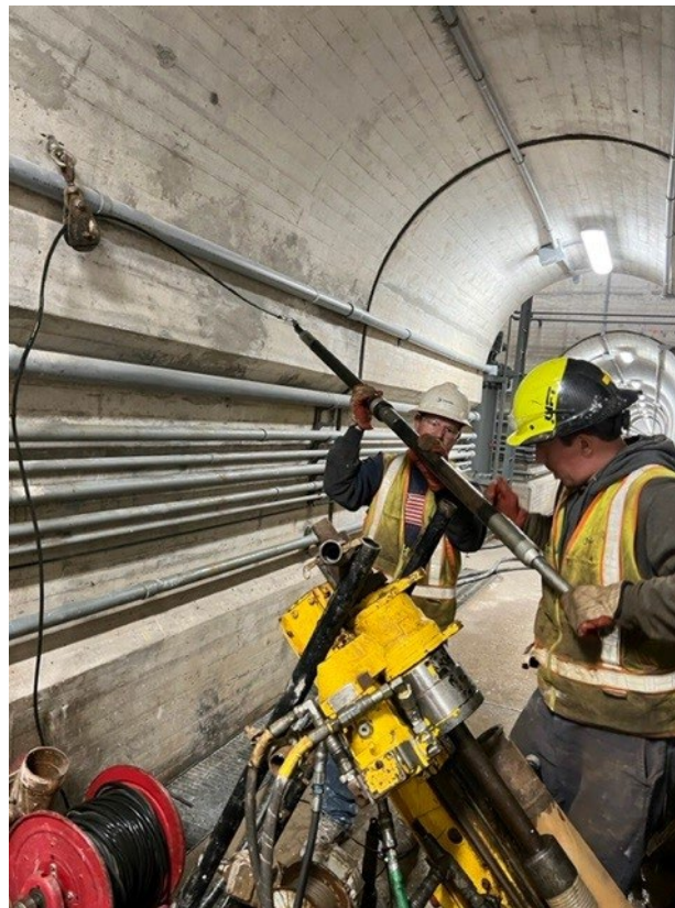
Figure 8: Vibrating Wire Piezometers installed in the operating gallery of John Martin Dam.
