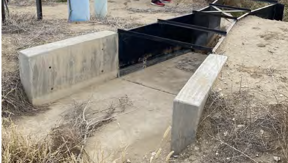
Figure A7 ARF27LCO flume profile with waterline (facing downstream)
