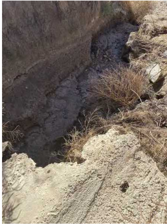
Figure A25 Wheatridge Augmentation Station Downstream Undercutting
