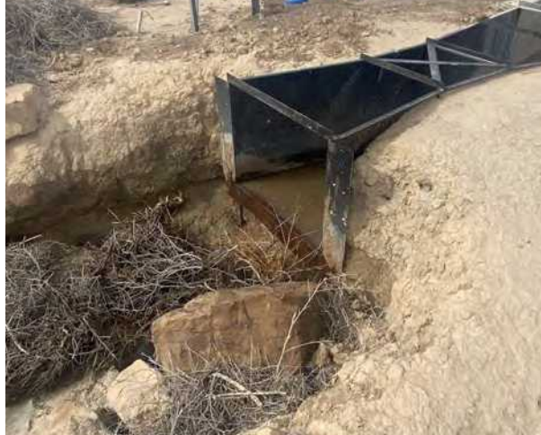
Figure A20 Farm 65 Inlet Flume Downstream outlet
