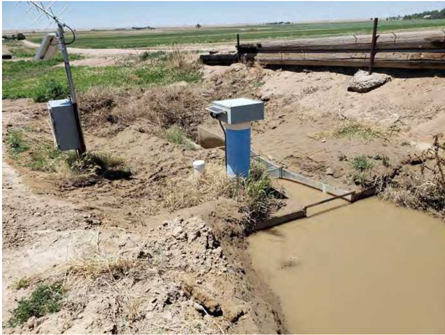
Figure A29 Farm 110 Recharge Facility Measurement Device
