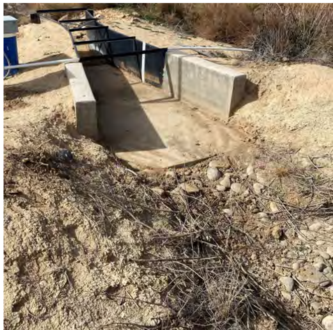
Figure A23 Farm 65 Downstream Augmentation Station (ARF16TCO) Upstream flume stilling pool
