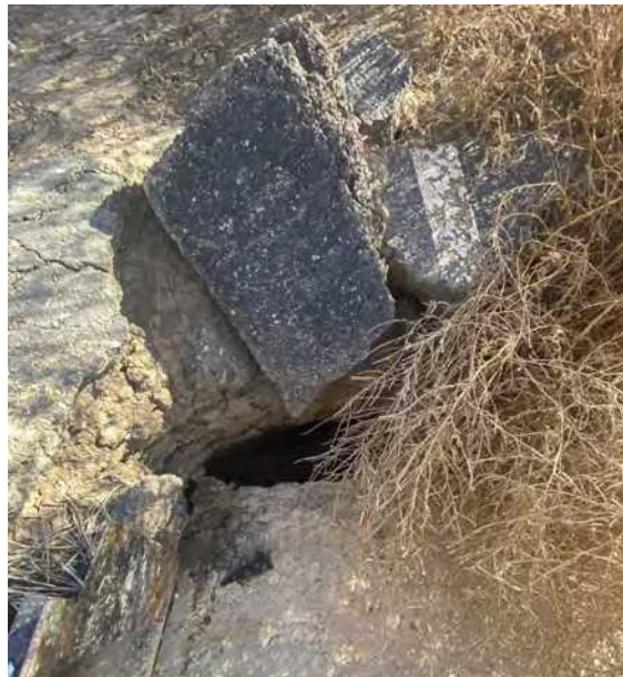
Figure A26 Wheatridge Augmentation Station Downstream Sidewall Erosion
