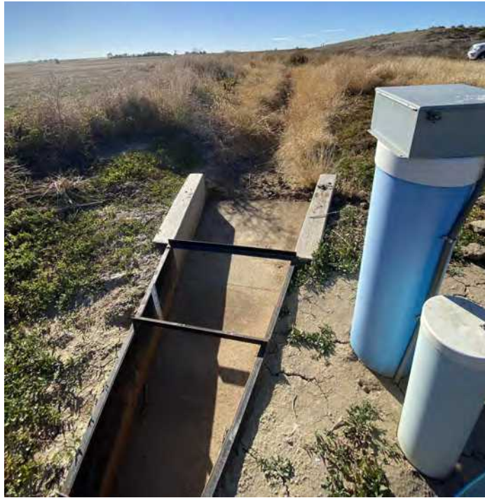
Figure A36 Farm 110 Storage Facility Channel between the Storage Ponds and Lower Augmentation Station
