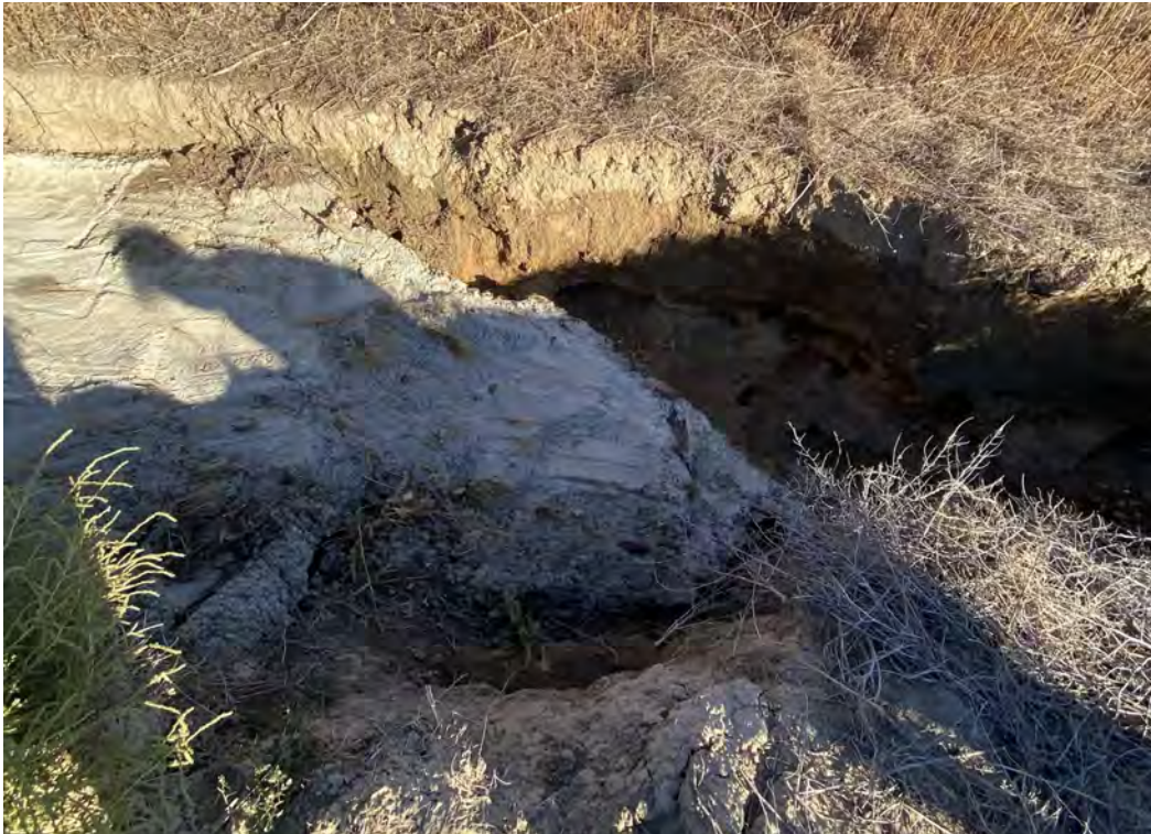
Figure A39 McClave Augmentation Station Downstream Erosion and Undercutting
