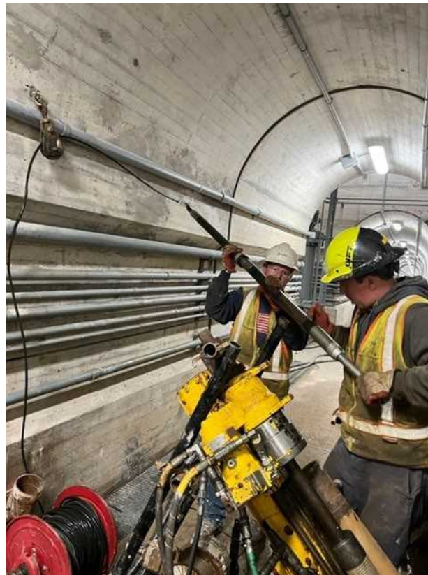
Figure 8: Vibrating Wire Piezometers installed in the operating gallery of John Martin Dam.
