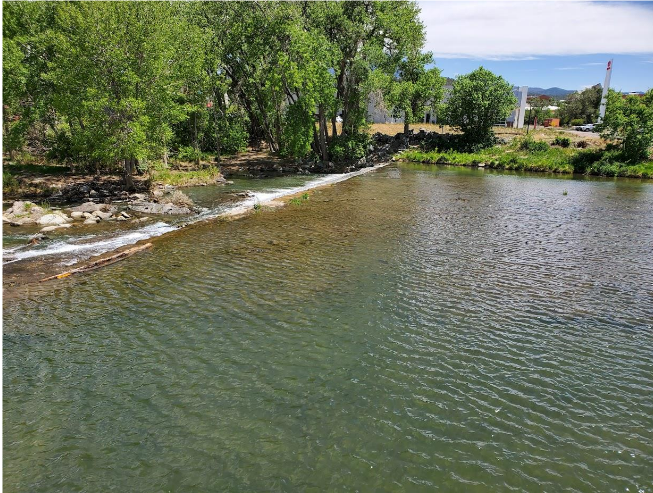
Picketwire/Baca Ditch Diversion Dam area with “Island” removed (March 2022). Dam still in deteriorated condition.
